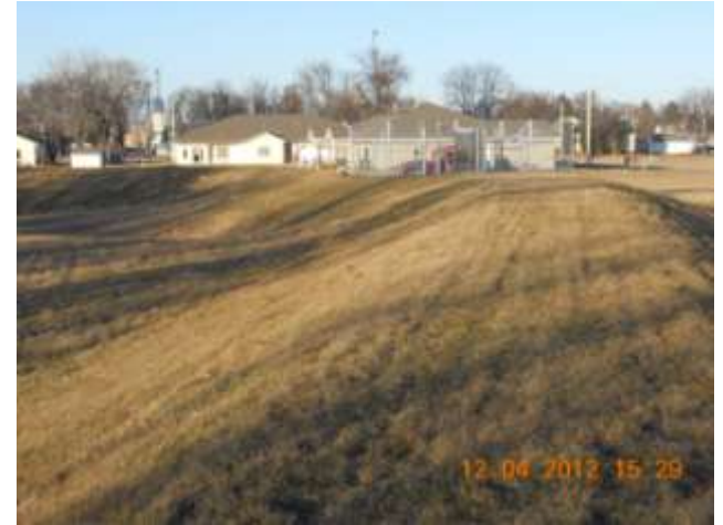
Near Buffalo Ave. & 3 rd St. S. in Breckenridge, MN Height: 4-5 ft, Side Slopes 1:3
